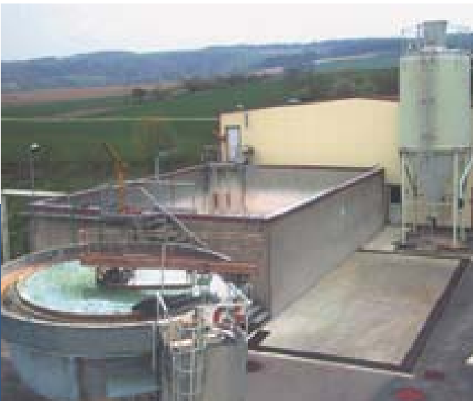
Industrial-waste plant at the Ligny en Barrois (Les Battants) factory in France
